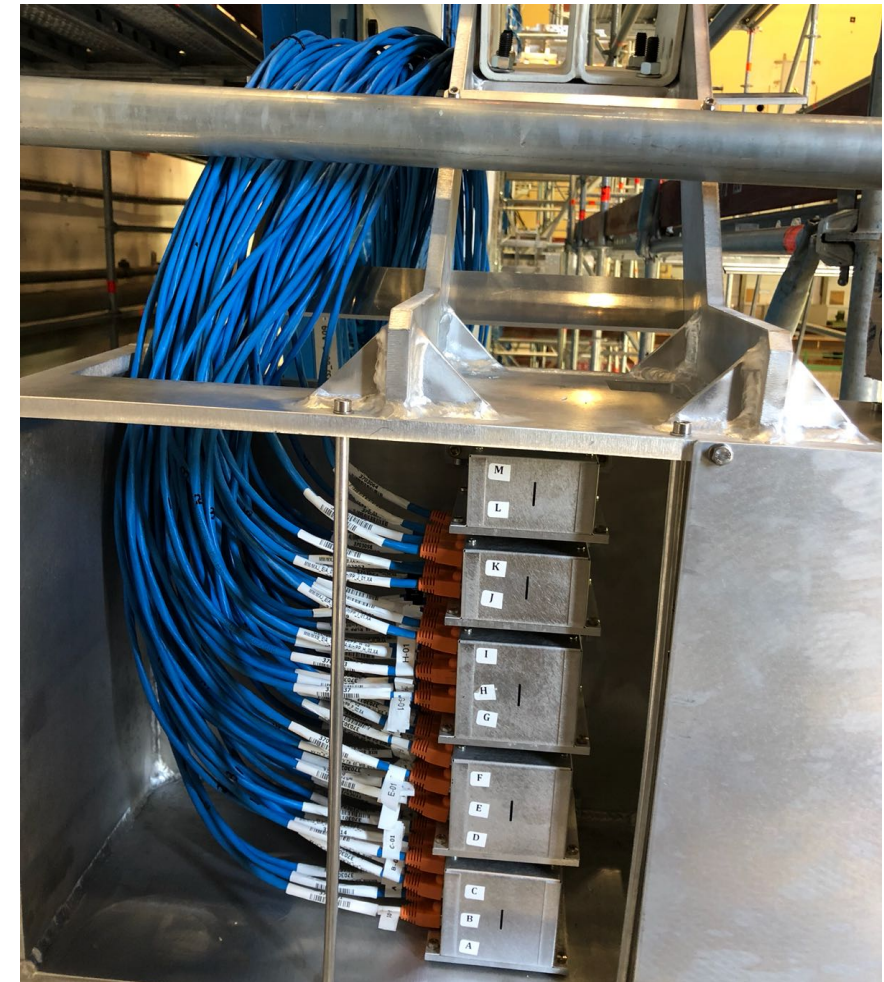
Alignment root cables and repeaters in A-side patch panel
